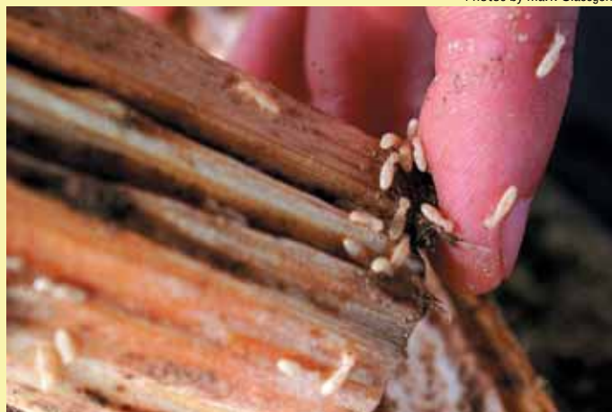
When the crates used in the research project are dug up, the soil and wood inside are filled with Formosan subterranean termites.
