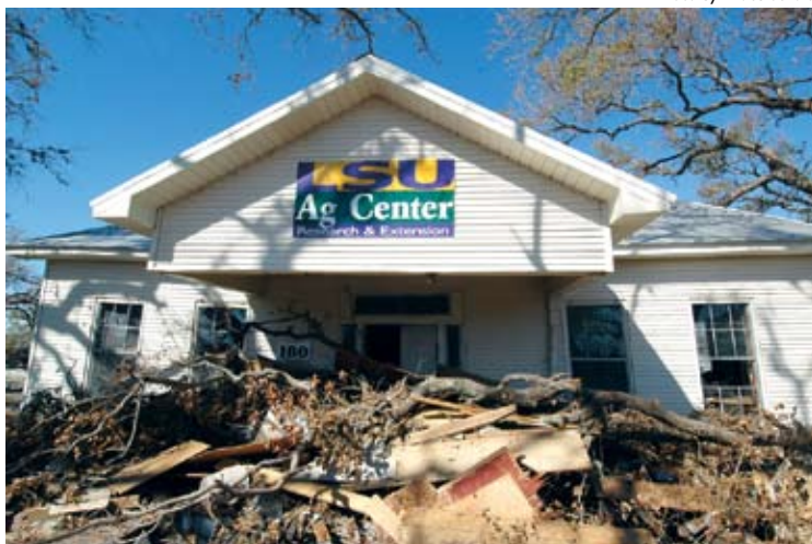
The Cameron Parish extension office was swept off its foundation by the surge from the Gulf of Mexico during Hurricane Rita on September 26.
