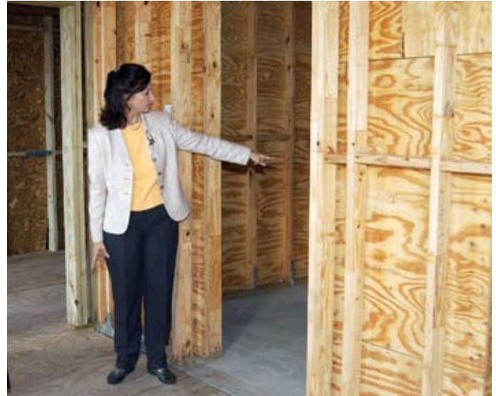
Claudette Reichel shows where the steel pocket door would protect occupants of the safe room if they were to use it to escape the threats of high winds or intruders.
