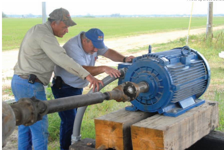
Farmer Neal LeJeune of Duralde, at left, and Keith Fontenot, LSU AgCenter county agent in Evangeline Parish, look at a new 200-horsepower electric motor installed on a well at LeJeune's farm to pump 4,500 gallons a minute. LeJeune said a new diesel replacement engine would have cost $18,000, he said, compared to the $14,500 cost of an electric unit. The operation cost will be $320-380 a day, compared to $856 a day for diesel at $3.57 a gallon.
