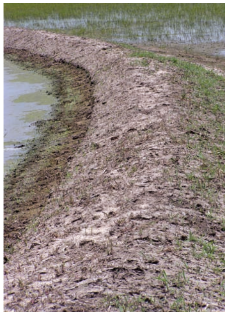
Note the lack of vegetation on the left side and top of the levee. The vegetation was killed by drift of the herbicide Newpath with the predominant wind traveling from left to right in this picture.
