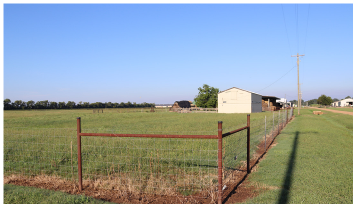
Pipe H-brace/corner. Photo by Abby Dunn
