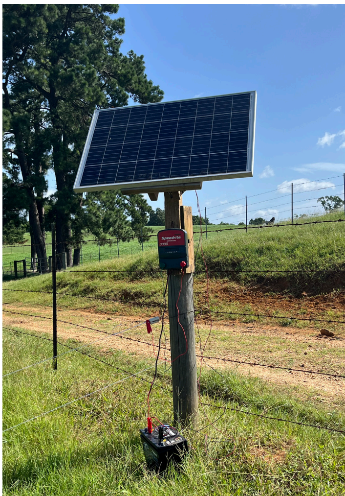
Solar power may be used to provide energy for an electric fence. Photo by Tripp Morgan
