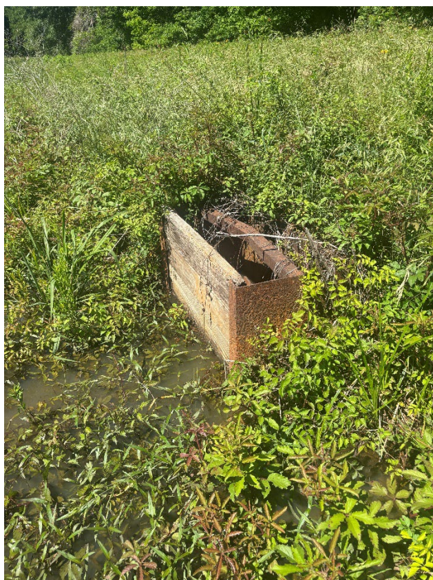
Figure 1. Water control structure placed in levee of moist soil unit to manipulate water levels.
