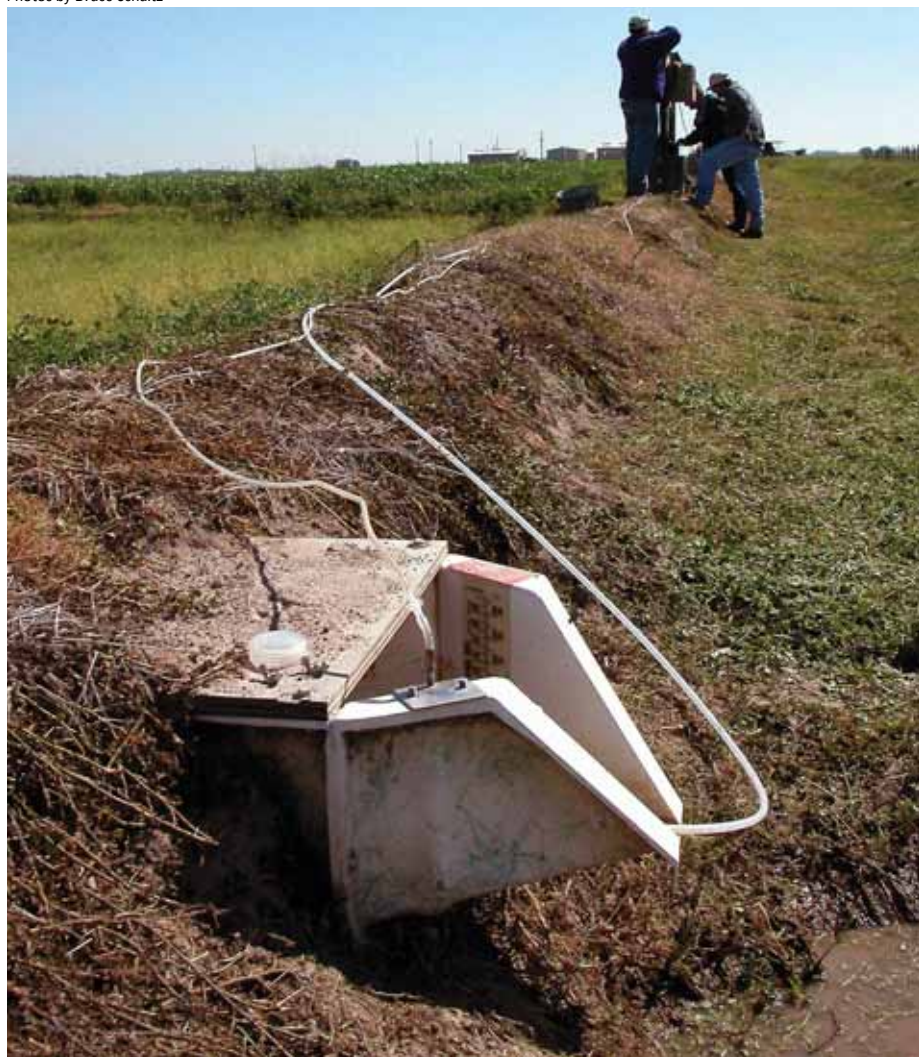
This H flume is installed in a levee surrounding a soybean field at the South Farm of the LSU AgCenter's Rice Research Station, Crowley.
