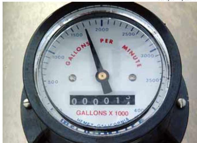
A flow meter inside this delivery pipe stationed in Beauregard Parish gathers data on water use throughout the growing season.
